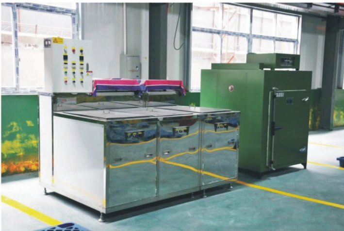
脱脂装置 Degreasing Plant
